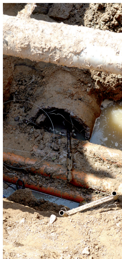
污水管被顶破
